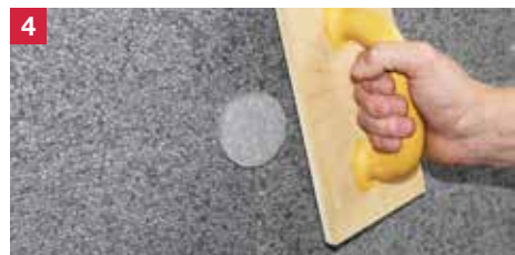
Using a float, or flat object to insert the ejotherm STR insulation cap flush with the surface - ready
